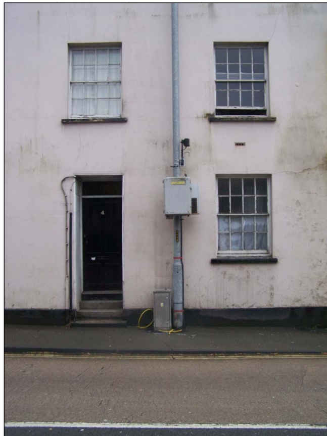
Plate 1. The airpointer ® in Dennison Road (with MOVA antennae installed above).
