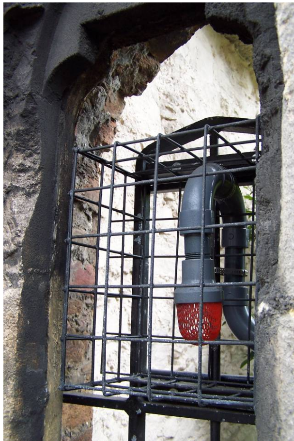
Plate 3. The inlet head for the monitor situated in a recess viewed from Penryn Street.
